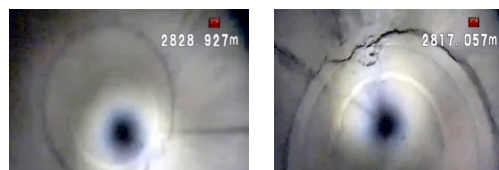
图1 可视化测井变形套管和套管未变形接箍对比 Fig. 1 Comparison of collar of deformed casing and undeformed casing in visualized logging
